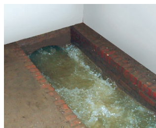
Downsurge flush in inverted siphon
