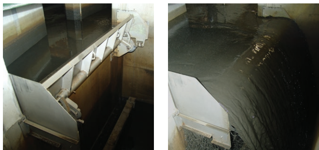
HydroBend Weir Gates in sewer, no external energy
